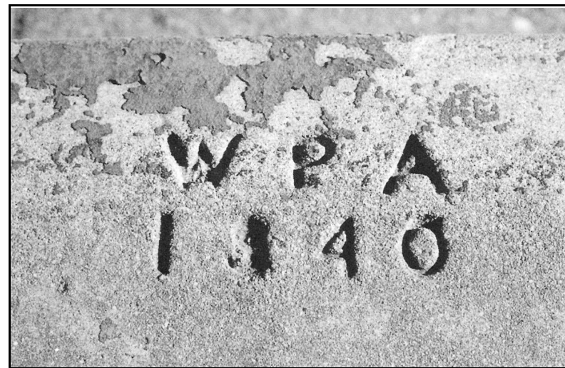
WPA was responsible for the installation of many curbs such as this one.
